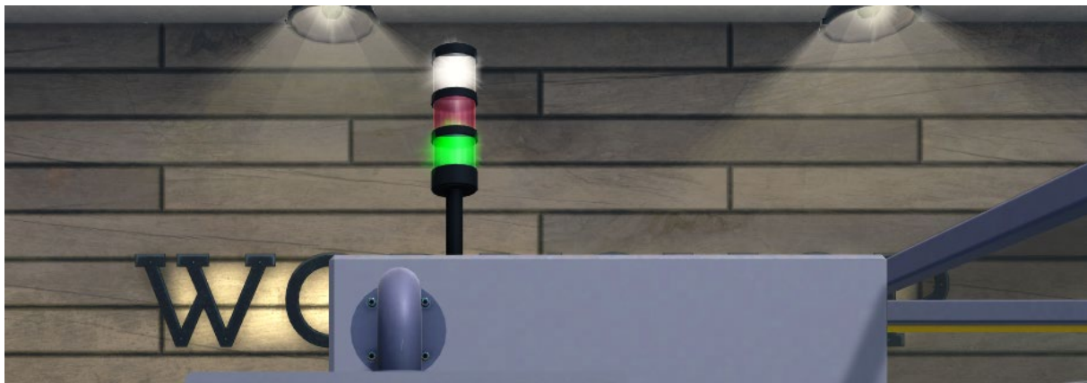
Figure 20 – Indicator lights when the machine works properly
